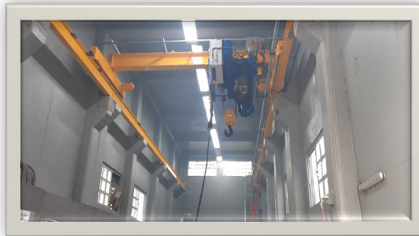
New Overhead Crane for Use on Pump Maintenance
