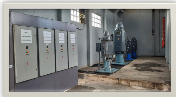
Control Panel and Pumps
