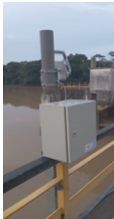
Water level sensor on a hydroelectric dam
